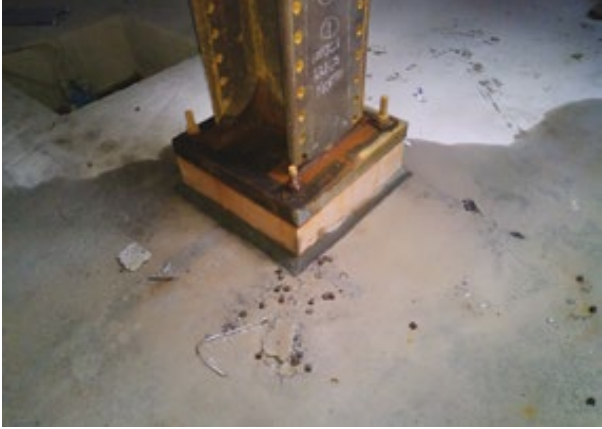
The beige color in the column base is 6-inch thick structural thermal break foam. This product’s compressive strength is higher than the concrete it sits on.
